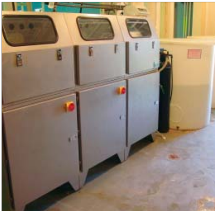
MIOX-252 system at Cedar Knox Rural Water Project.
