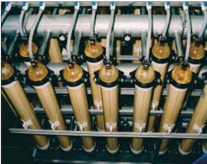
Visible here are the clear domes of several of the 36 UF cartridges at Cass County. The domes help with visual monitoring of fiber integrity.
