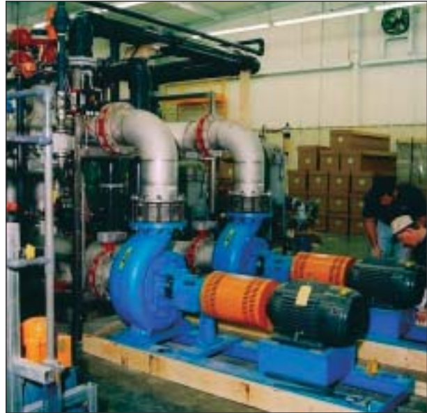
Shown here are two recirculation pumps for the UF cartridges, one of which is on standby to provide the redundancy required by state regulations.
