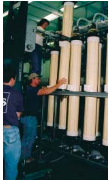
Installation of six-ft long, eight-in. diameter UF pressure cartridges on the system rack at Cass County.
