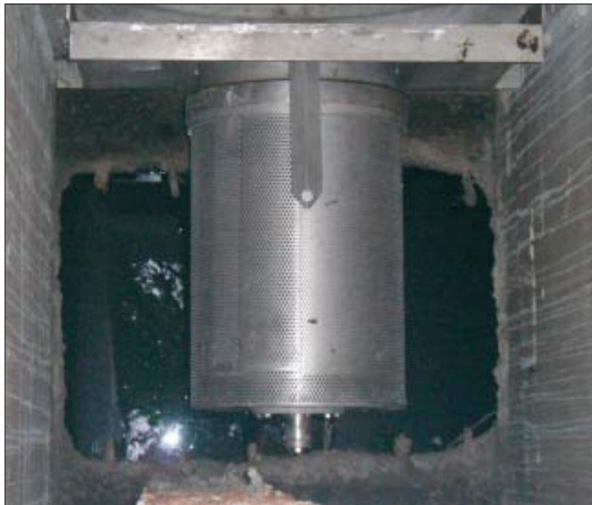
The perforated drum has 6-mm diameter openings, which remove all but the smallest gross solids from combined wastewater.
